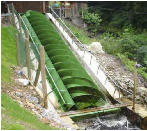
Source: The New England Hydropower Company Figure 1-8. Archimedes screw for hydropower generation
