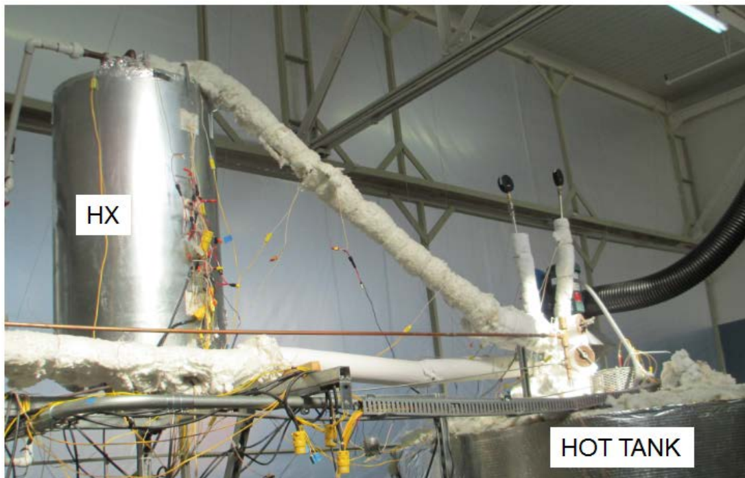
Figure 40. The HX is installed, plumbed, and electrical connections are made to the Hot Tank.
