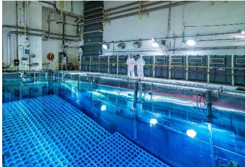
FIG. 1. Krško NPP Spent Fuel Pool (reproduced from Ref. [1] with permission).
