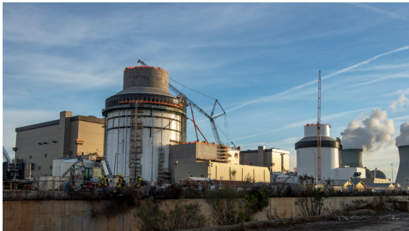
Units 3 and 4 of the Vogtle plant, pictured last month (Image: Georgia Power)
