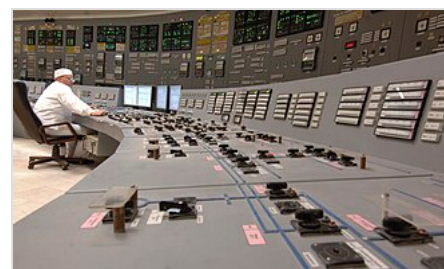
The control room of a first generation RBMK at Kursk Nuclear Power Plant
