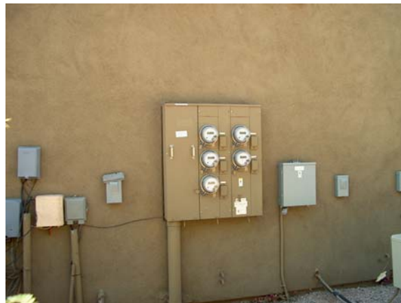
Figure 5-15. Typical apartment electrical distribution point.
