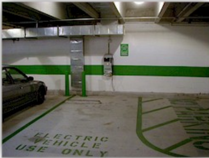
Figure 5-9. Example of ground striping for an Americans with Disabilities Act-compliant electric vehicle station.
