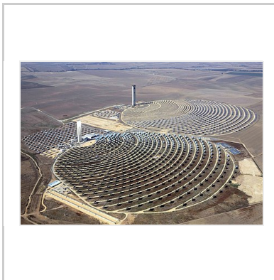
The PS10 and PS20 solar power plant near Seville, in Andalusia, Spain.
