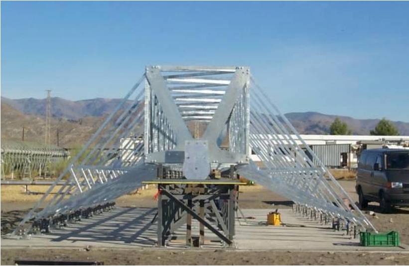
Figure 23: Assembly of the Eurotrough module with the help of an assembly jig (source: Lüpfert, DLR)
