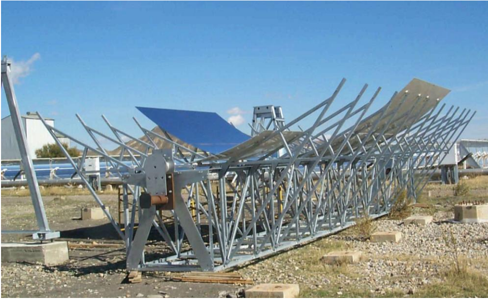
Figure 21: Space frame structure of a Eurotrough collector module (source: Lüpfer, DLR)
