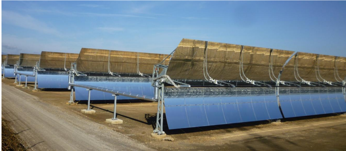
Figure 65: Connection of two collector rows to one loop (source: Simon Csambor)
