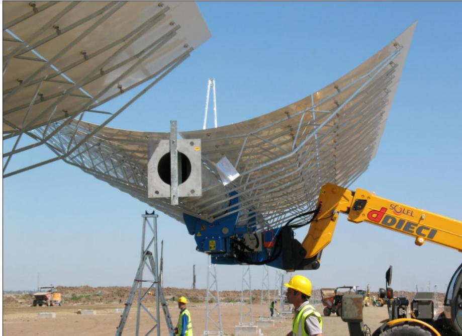
Figure 35: Siemens/ Solel Collector installation in Lebrija, Spain (source: Siemens)
