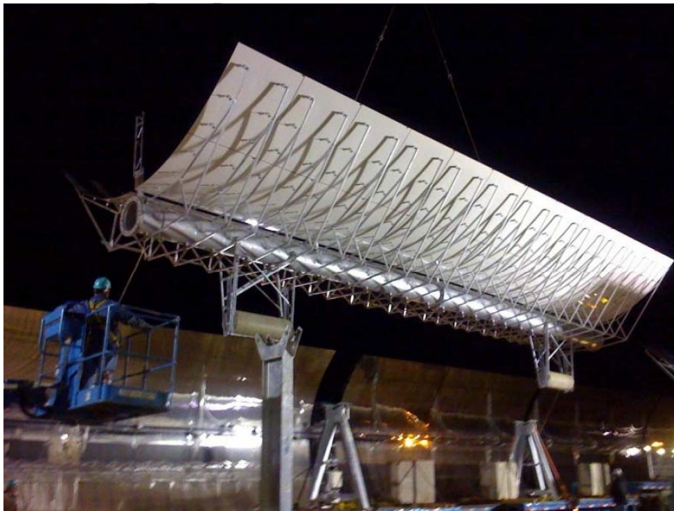
Figure 33: Installation of a Heliostroph collector element in one of the SEGS plants (source: Flagsol)
