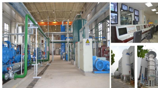
Figure 13. 1.5 MW SC-CAES pilot plant in China [60].
