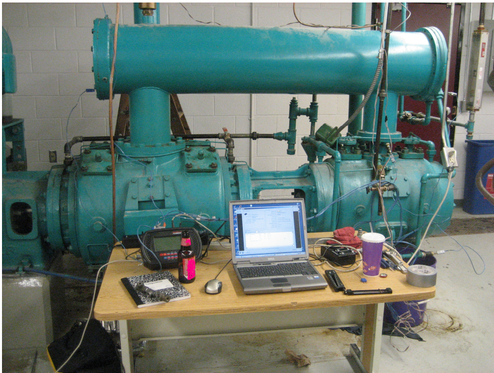
Figure 3-1 Gardener-Denver tandem horizontal two-stage compressor model RL 1155CB.
