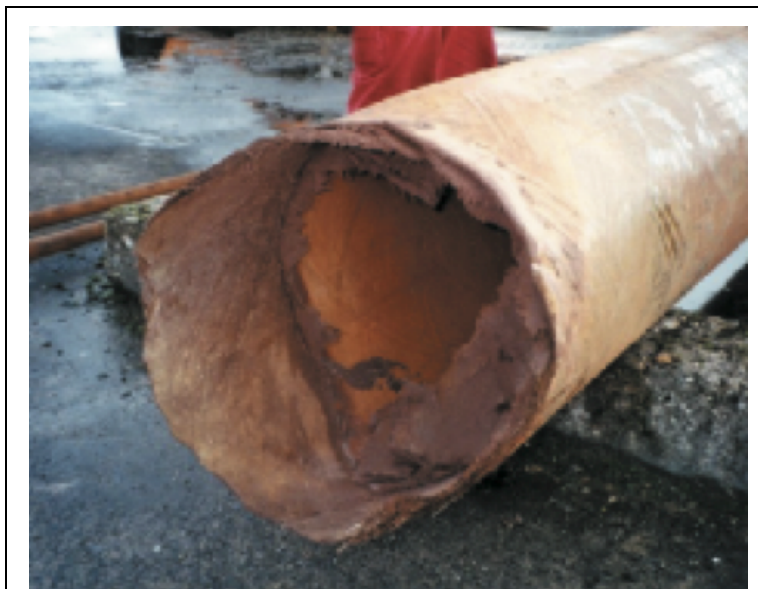
Figure 22 This photograph, from the Huntorf CAES facility in Germany, shows where the protective fiberglass-reinforced plastic tubing fractured. [35]
