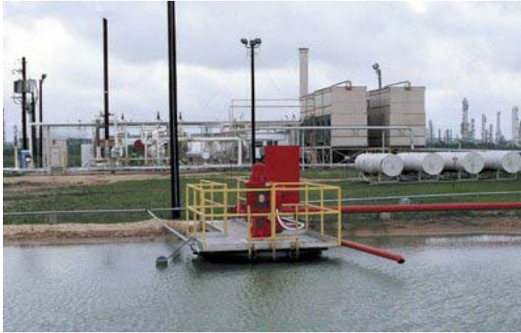
Figure 16: Geopressed Demonstration Plant in Texas
