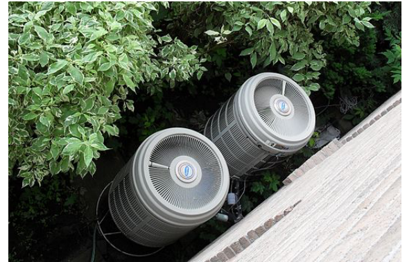
Outdoor components of a residential air-source heat pump
